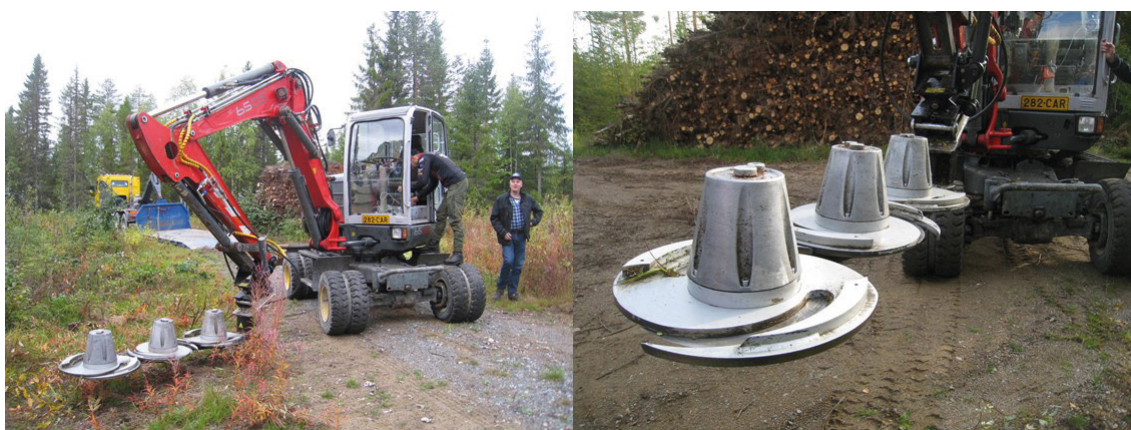
Fig. 2. JAK SP-180 spiral cutter was attached to the boom tip of wheeled Neuson 6503 WD mini-excavator. The clearing of brushwood was done with the spiral cutter in the study.
