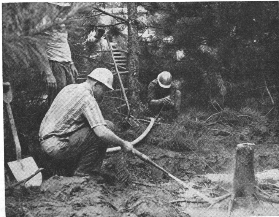
Figure 2. Excavation of the root system of red pine by means of a hydraulic jet of a 2,000 gallon capacity.
